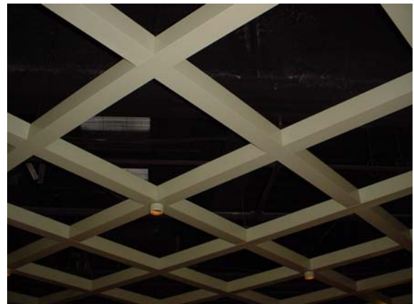
Figure 3 – Open Grid Ceiling
