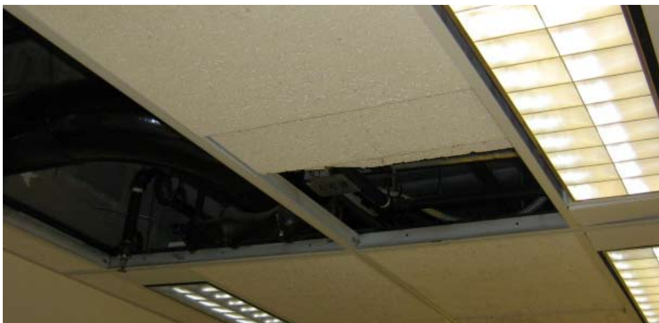
Figure 1: Missing and damaged ceiling tiles
