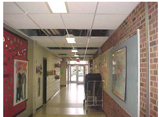
Figure 1 - Missing Ceiling Tile
