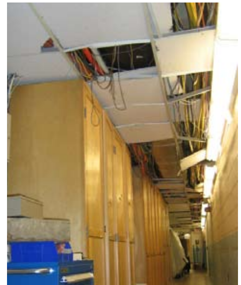
Figure 2: Removal of ceiling tiles may damage wiring to detectors mounted below them.
