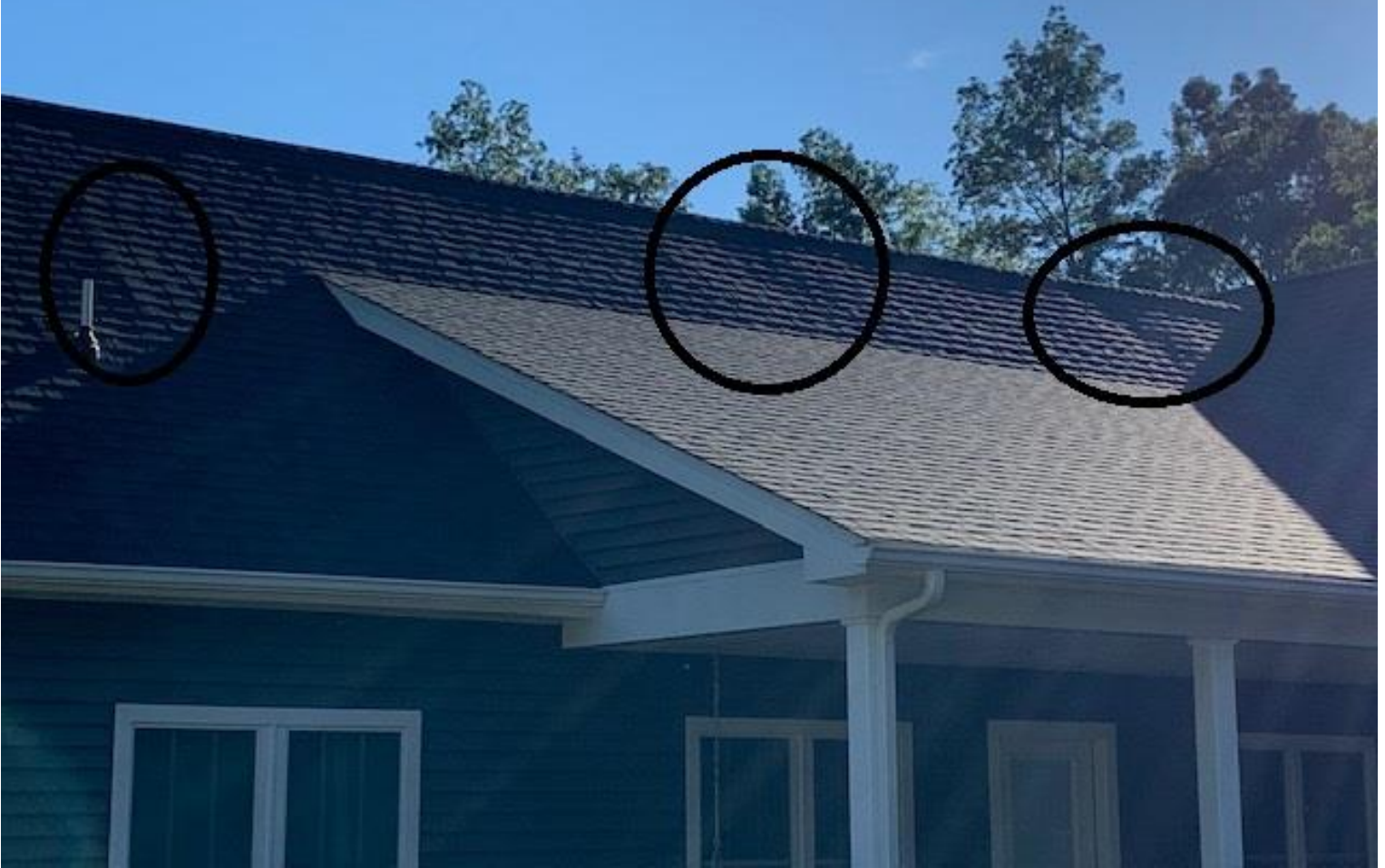
image taken by monica davis trusses raised higher causing sags in roof
