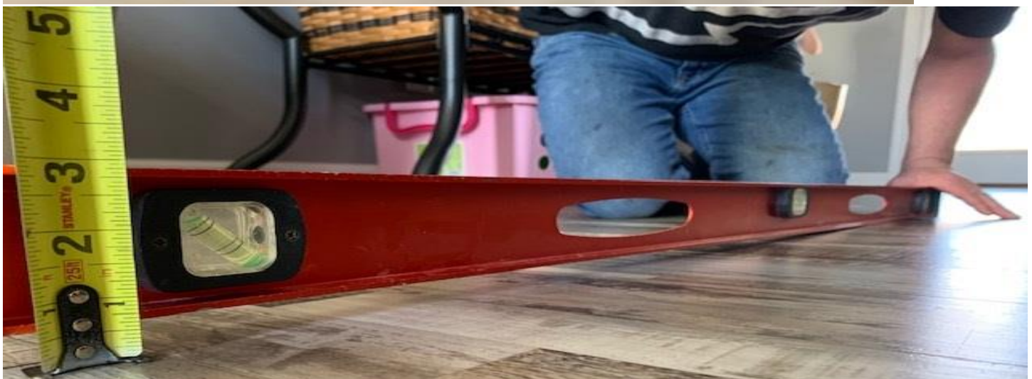
Image taken 2/16/21 by Monica Davis @ 11:56 AM. As indicated would happen by simpson literature due to the gape in the hangers and the improper hardware Joist with gap puts downward force further from header and creates more rotation. This image shows the location in the living room where the floor has dropped 5/8th of an inch
