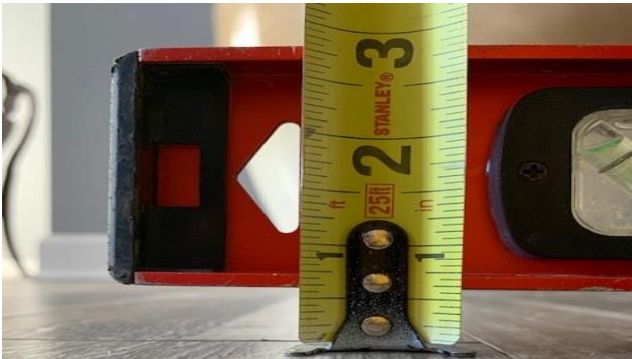
Image taken 2/16/21 by Monica Davis @ 11:56 AM. This image shows the tape measure close up in the location in the living room where the floor has dropped 5/8th of an inch
