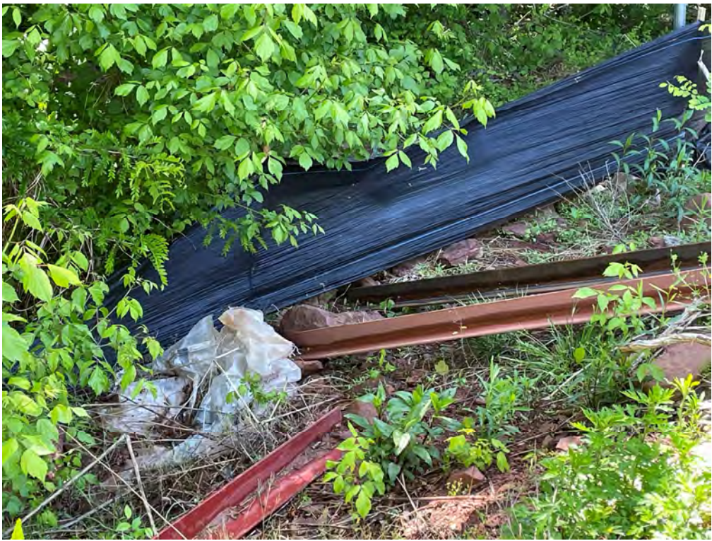
Incorrectly installed super silt fencing, not trenched in at bottom
