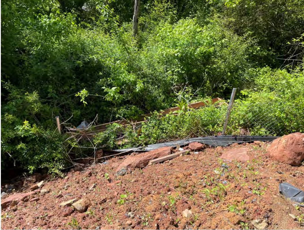
Unmaintained/ineffective super silt fencing, construction debris outside limits of disturbance in tree protection area.
