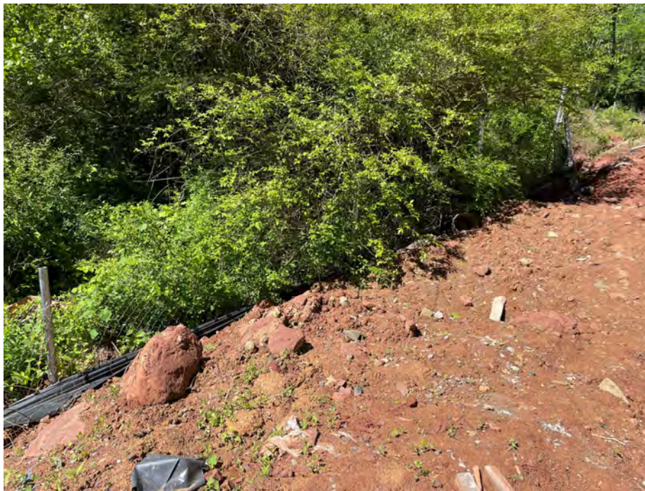
Unmaintained/ineffective super silt fencing
