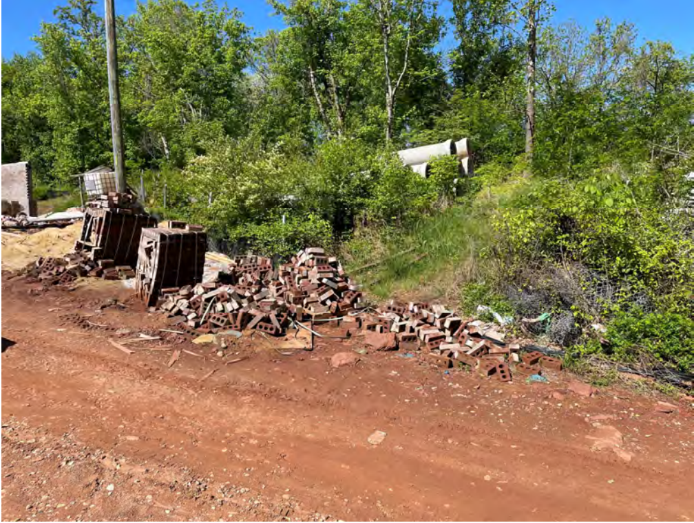
Damaged/uninstalled super silt fencing
