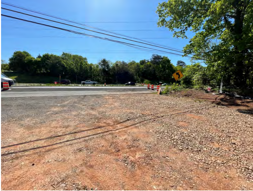
Ineffective construction entrance
