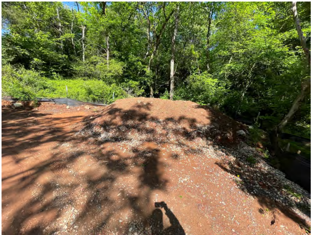
Stockpile not stabilized or protected
