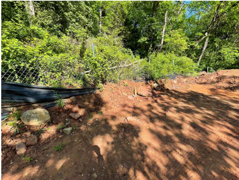
Unmaintained/ineffective super silt fencing
