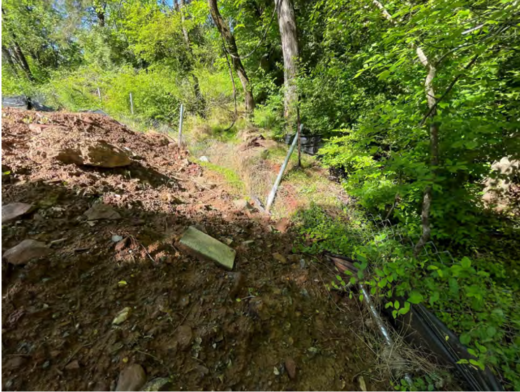
Unmaintained/ineffective super silt fencing
