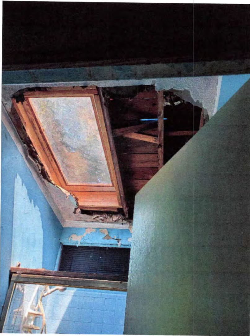
Figure 2 – Hall Bathroom Ceiling
