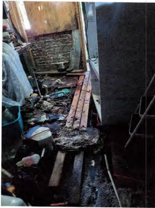
Figure 5 – Kitchen Floor Damage
