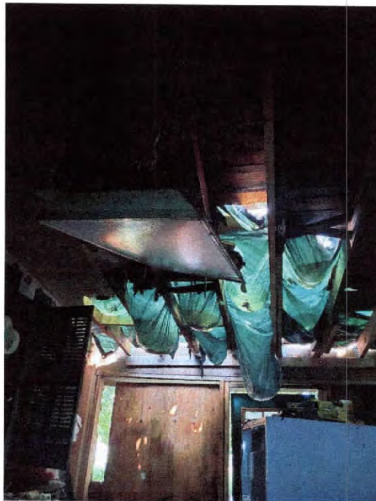
Figure 4 – Kitchen Ceiling/ Wall damage
