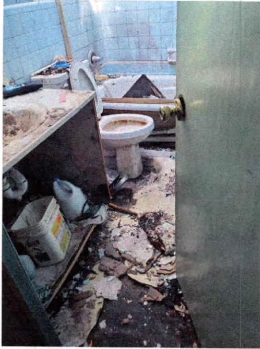
Figure 3 – Hall Bathroom Floor
