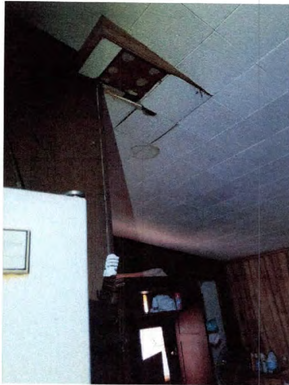
Figure 7– Ceiling Damage Example
