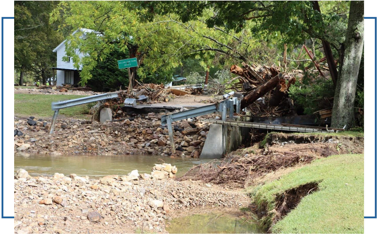
Figure 5: Destroyed Bridge in the City of Bristol
