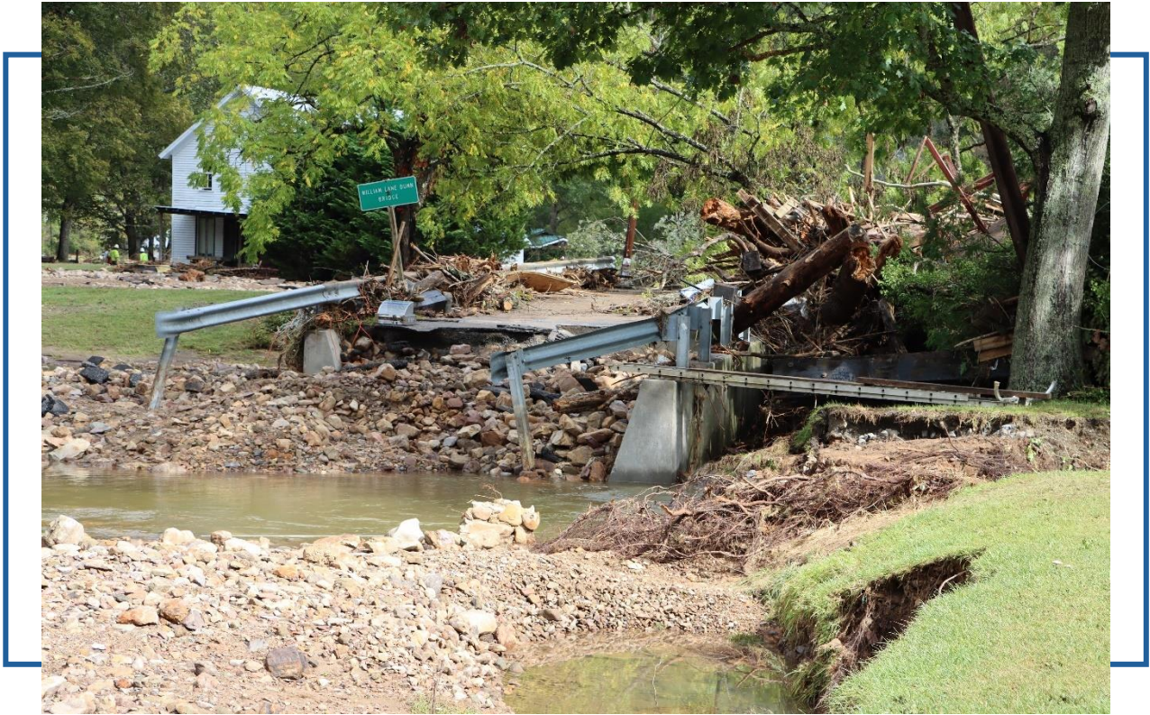
Figure 5: Destroyed Bridge in the City of Bristol
